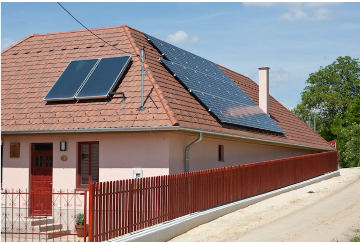
Picture 1: 6.56 kWp photovoltaic solar system (right) and solar collectors (left) at the Middle House.
